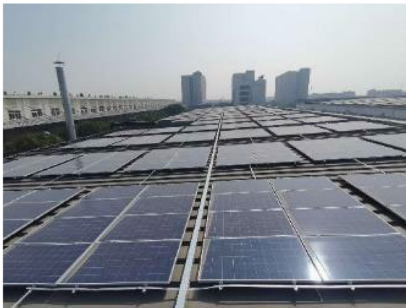
Solar panels newly installed on the roof of Fujitsu General Central Air-Conditioner (Wuxi) Co., Ltd.
