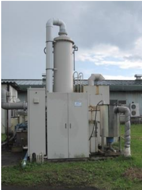
Groundwater purification facility (Aomori Business Office)
