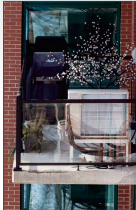
Outdoor condensing units sat on patios for each individual condo unit. There were a total of 79 systems installed in the condo development overlooking a finger of Halifax Harbor.
