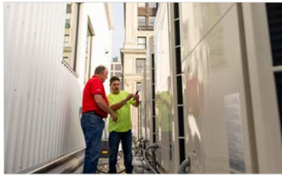
Alan Dukes (left), of Ferguson Enterprises, and John Jenkins, assistant supervisor at Snyder Solutions, discuss the Fujitsu Airstage heat recovery installation on the roof of the Mutual Building.
