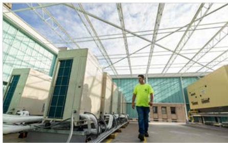
John Jenkins, assistant supervisor at Snyder Solutions, walks the rooftop of the Mutual Building.
