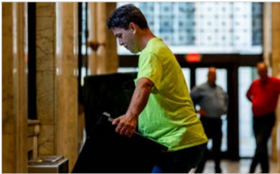
John Jenkins removes wooden casing from around a vertically-mounted Airstage ARUL slim duct fan coil.
