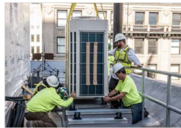
Airstage condensing units were mounted on seismic isolators.
