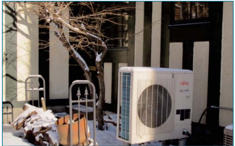
One outdoor condensing unit, AOU48RLXFZ1, was able to connect to the 4 indoor Slim Duct units.
